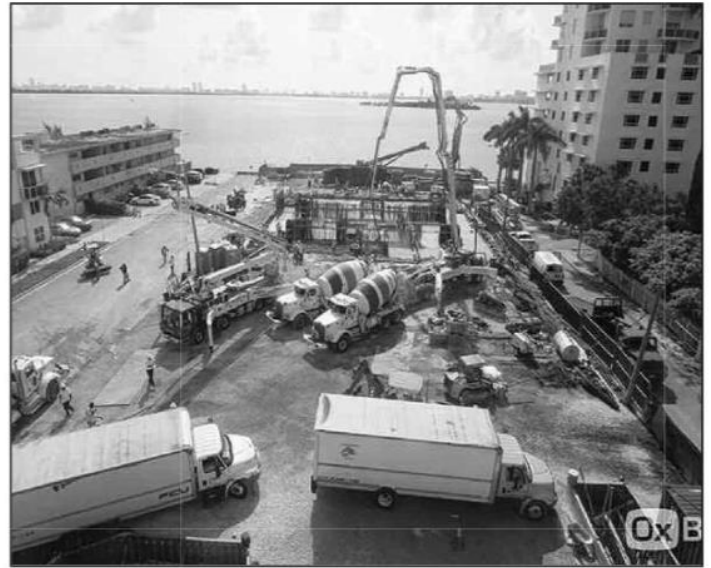
About 20 mixing trucks carrying 260 truckloads rotated in shifts to pour approximately 3,000 cubic yards of concrete weighing more than 5,000 tons.
